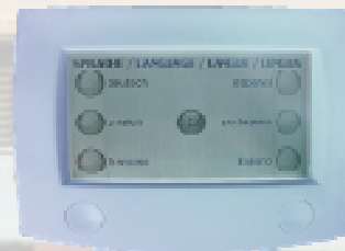
Energiemanagement Regeling SolvisControl2
